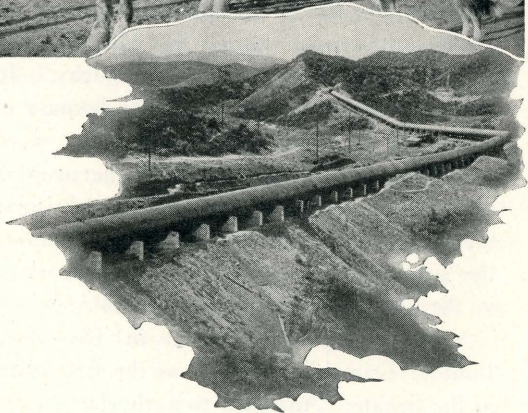
(Upper) Photograph taken twenty-two years ago, when Owens River Aqueduct was under construction, reveals the size of a section of Aqueduct siphon pipe. (Lower) Completed section of Aqueduct. The Colorado River Aqueduct will be almost four times larger in capacity.
