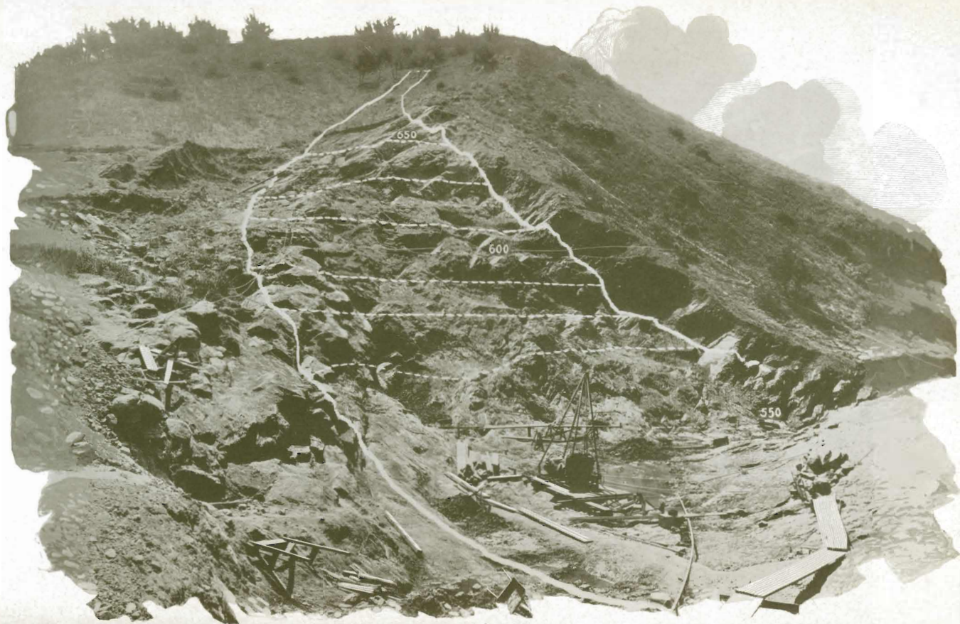
SECTION OF EASTERLY HALF OF STRIPPED SITE - HOLLYWOOD DAM, JUNE 1923 (DAM ITSELF WILL OCCUPY THE SPACE SHOWN BETWEEN THE WHITE LINES)
