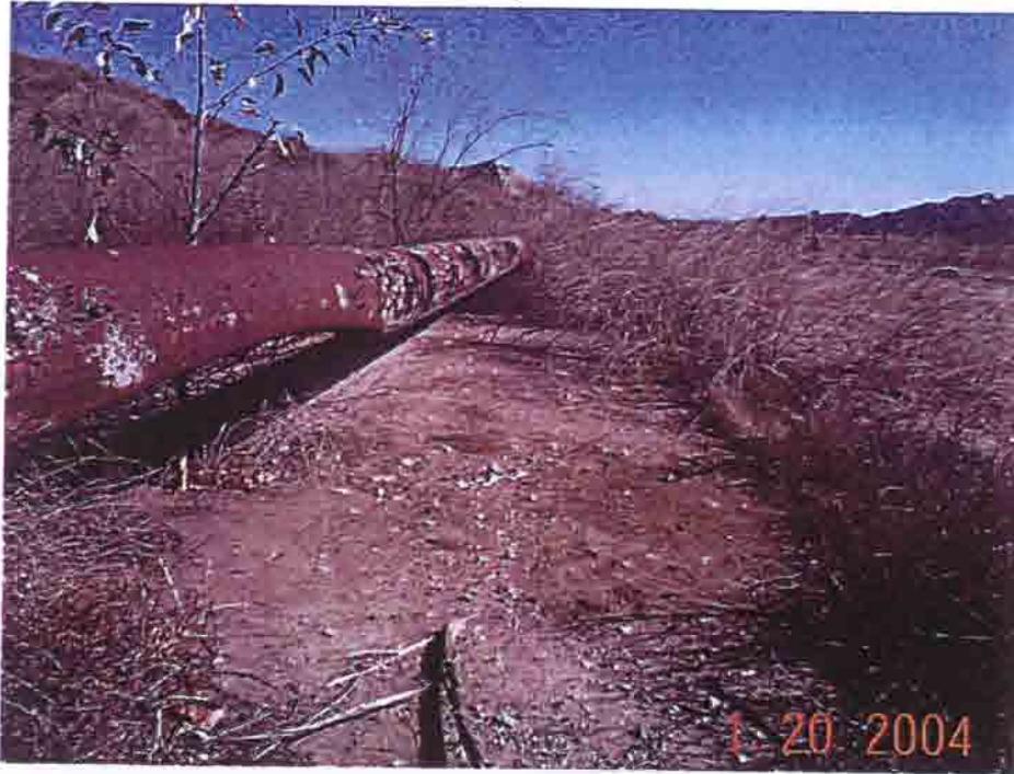
9. Exposed, abandoned oil pipeline. Note oil staining beneath pipe.
