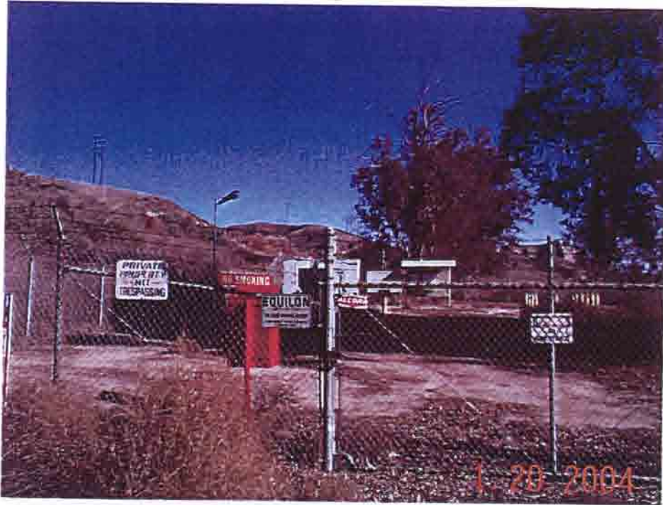
5. Booster station along pipeline easement, northern property boundary.
