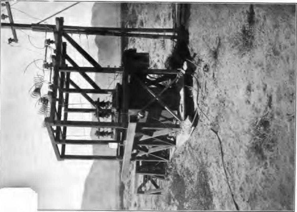
Outdoor Type of Transformer Used in Construction Work
