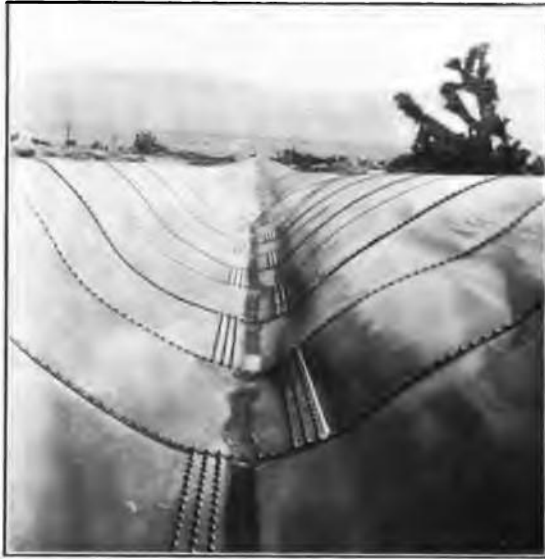
Collapsed Antelope Siphon
