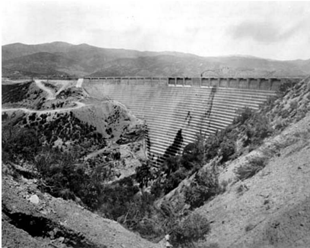
South face of the St. Francis Dam as it appeared just before the disaster on March 12-13, 1928.
