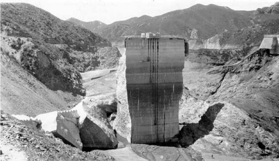
Inside of the destroyed St. Francis Dam looking southward.
