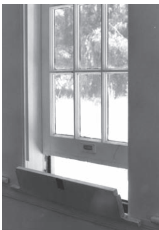
The cottages had unique sashes that lowered the window down into the wall
