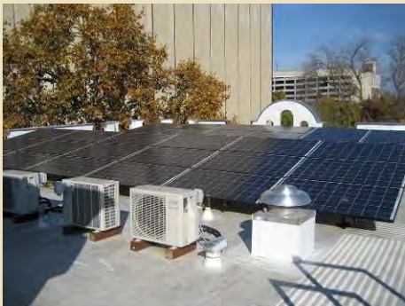
Low-profile photoelectric panels on the roof helped the building achieve LEED silver certification.
