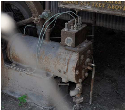
FM gas-fired engine showing spark plug, gas pipe, and electrical (?) box
