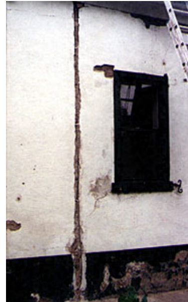
A vertical steel cable recessed into an exterior wall. The cable will be prestressed, then covered with adobe mortar.
