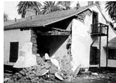
Two views of a section of Rancho Camulos, before and after the 1994 Northridge earthquake. Photos: Courtesy Shirley Lorentz.
