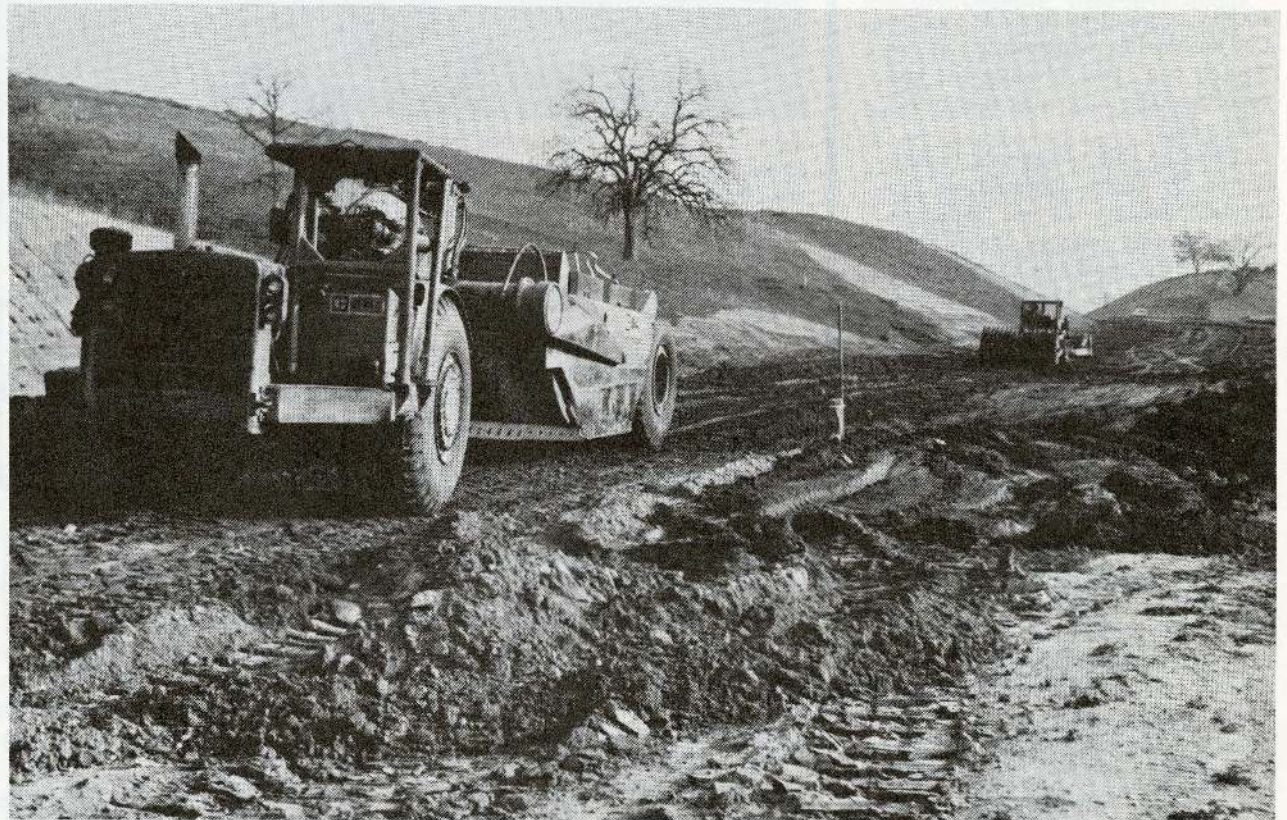
Heavy rains have slowed up work on the extension of Rockwell Canyon Rd. New thoroughfare, which will provide a southern entrance to COC, will be completed about 45 days after work resumes. The road, flanking COC on the east, will tie in Valencia Blvd. and McBean Pkwy. All the heavy earth movement is completed on project.
