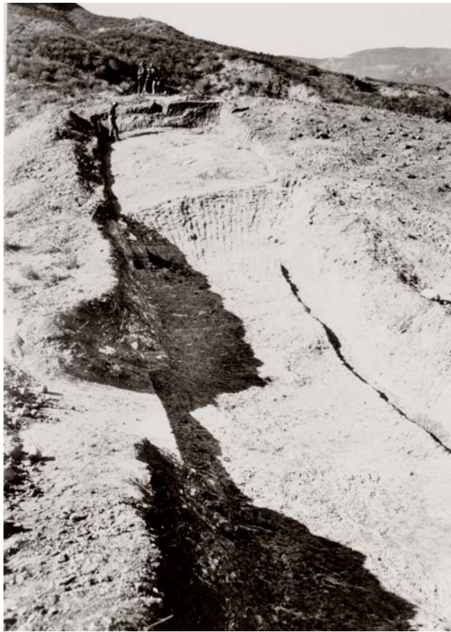
Figure 6. Keyway excavation in the Vasquez conglomerate cut by steam shovel for the dam's dike section, which extended about 600 feet northwest of the right abutment crest. Photo taken from Lippincott collection, U.C. Water Resources Center Archives.
