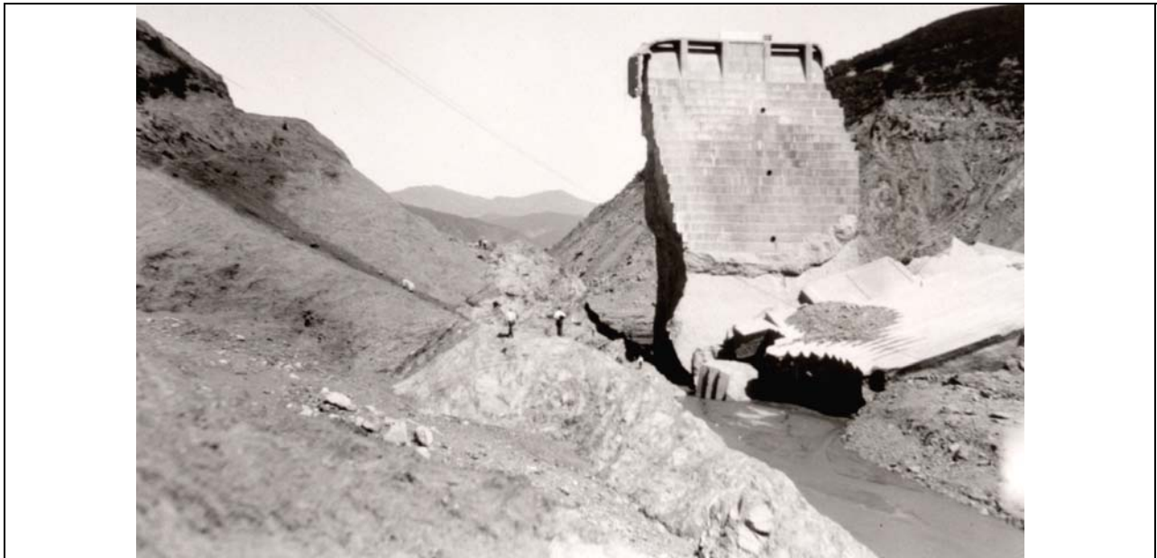
Figure 41. View of San Francisquito fault contact, between the Vasquez sandstone (at left) and Pelona schist (center of image), as viewed looking upstream at the dam's right abutment. Note the graphic nature of the contact, planed off by the outpouring water. Also, note the downed SCE power lines, trending towards the east abutment slide, out of view to the right. These lines were clipped before the Governor's Board of Inquiry visited the dam site (from Lippincott Collection of the U.C. Water Resources Center Archives).
