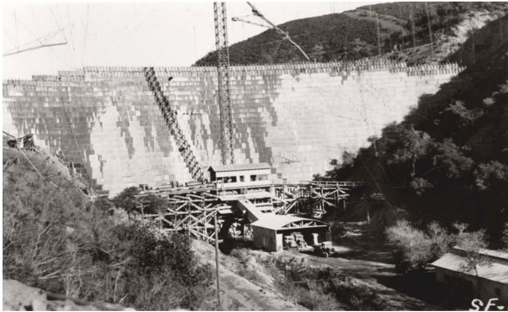
Figure 4 (Lower) - Same view as above, but about a year later, when the dam was nearing completion. Each of the steps were five feet high and forms can be seen along the upper three tiers. Note the dump trucks parked in the shed in front of the batch plant. Photo LA Dept of Water & Power.
