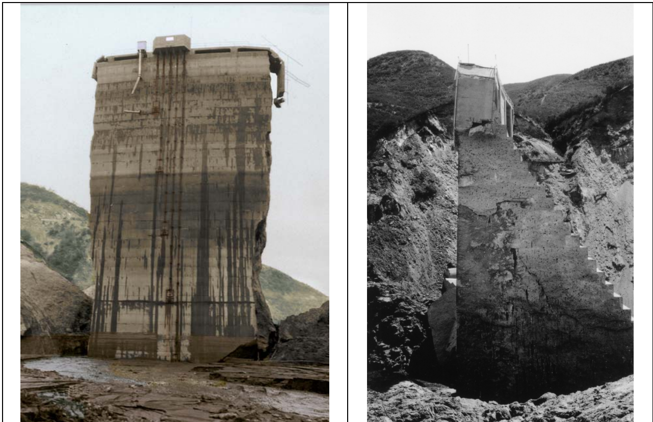
Figure 17. Left - Carl Grunsky discovered the gage attendant's wooden ladder wedged inside an enormous tension crack in the right upstream heel of Block 1 (from Ventura County Museum of History & Art; colorized by Pony Horton). Right - Profile view of the Block 1 monolith. No discernable upstream batter can be seen near elevation 1730, about half the height of the block (from La Rue Collection of the Huntington Library ).
