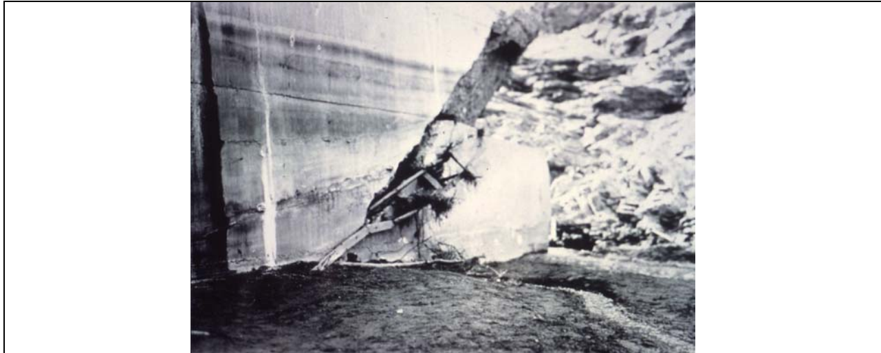
Figure 18. Detail view of the wooden gage attendant’s ladder found in a large tension crack in the right upstream heel of Block 1. This testifies to significant deformation of Block 1, tilting downstream under active hydrostatic pressure. Some of this may have occurred after Block 2/3/4 fell away, removing lateral restraint on the left side of Block 1. Photo taken from Outland (1963).
