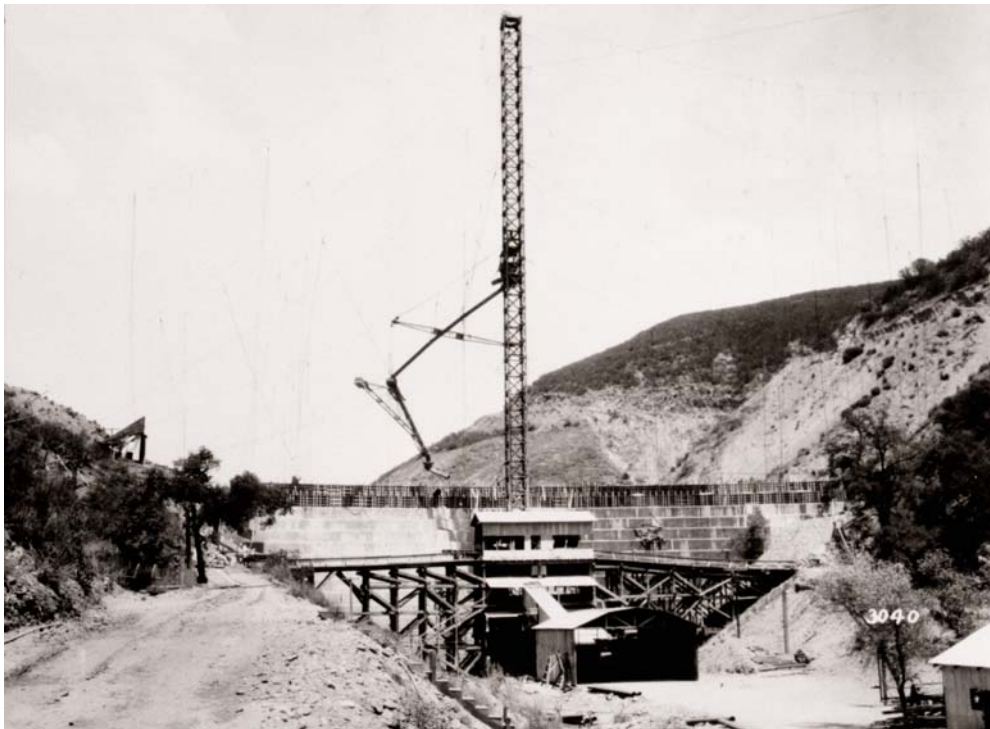
Figure 4 (upper). Upstream view of St. Francis Dam under construction, in the fall of 1924. The contractor’s concrete batch plant lies in front of the dam. The large shed in front of this structure was where aggregate collected down-canyon was end dumped into the plant. Photo from the Lippincott collection, U.C. Water Resources Center Archives.
