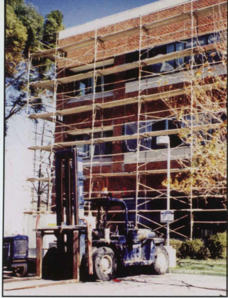
City Hall was severely damaged during the earthquake and was subsequently repaired and retrofitted.
