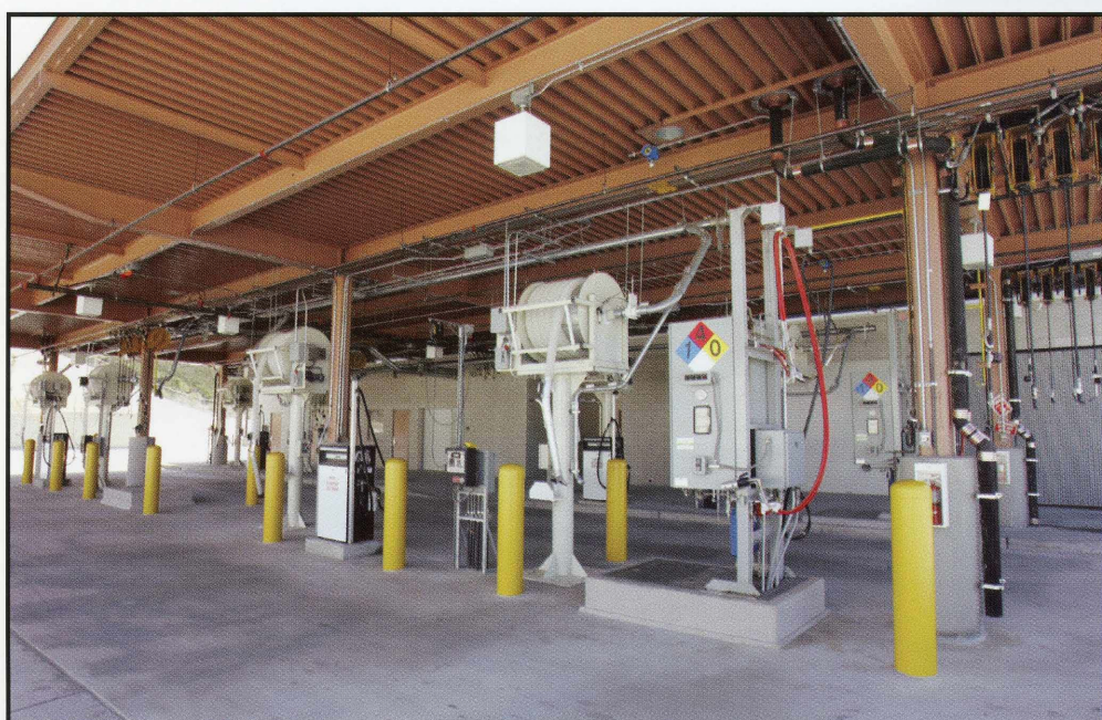
The Transit Maintenance Facility in the Valencia Industrial Center opened in 2006 and provides a central location for the City's transit fleet. Pictured here: bus wash area.
