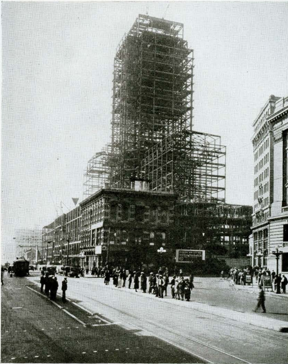
The last stand of the historic Temple Block. As the steel frame of the new City Hall neared completion the proud old building, once dominant in the business and professional life of the city, was razed
