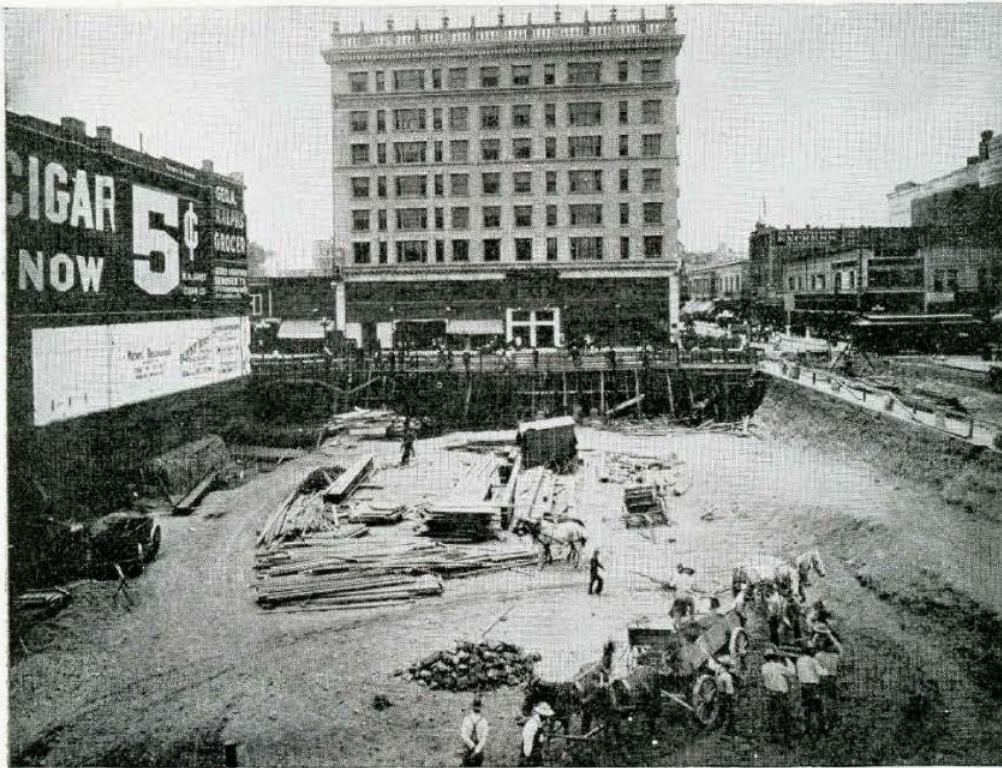
When the excavation was made for the Security Building in 1906 the Alexandria Hotel had just been completed
