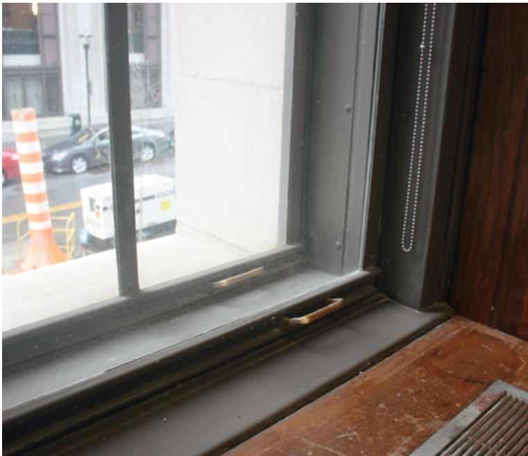
[18] The historic metal storm windows in this 1920s office building were retained and repaired during the rehabilitation project.
